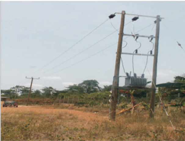
Connection to the National Grid
