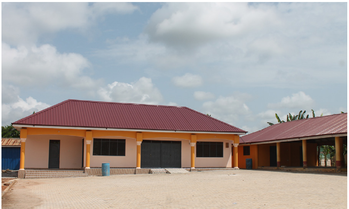
Pictures 20: Construction of Conference Hall and an out house at Mamanso durbar ground
