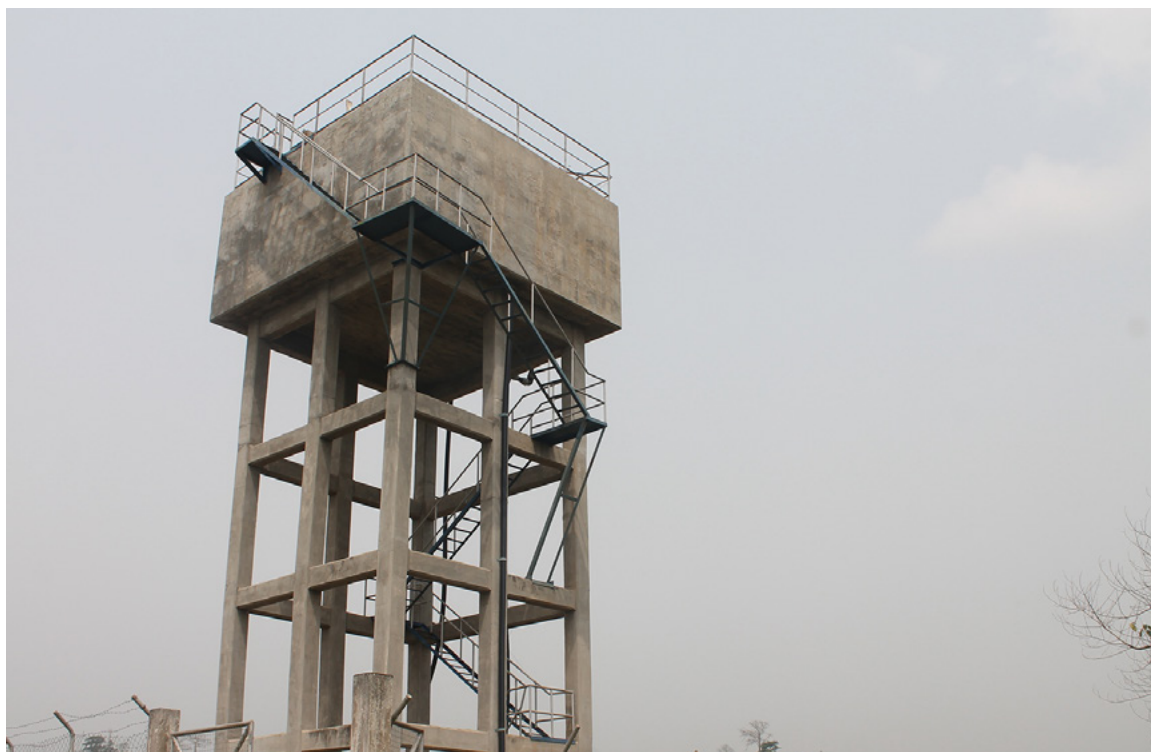
Picture 18: Construction of Hweakwae/Adausena high level water tank Retaining wall and chain link fencing
