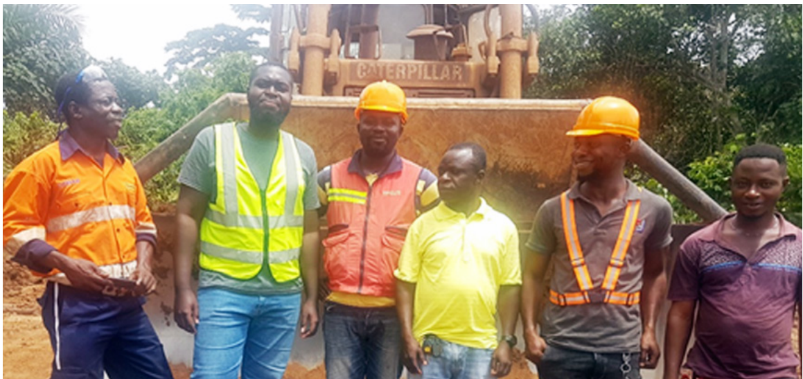
Picture 19 - Construction of access road to Oil Palm Plantation for the Resettlement community at Kyenkyenku
