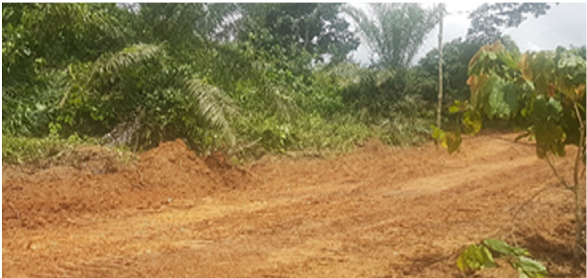
Picture 18 - Construction of access road to Oil Palm Plantation for the Resettlement community at Kyenkyenku
