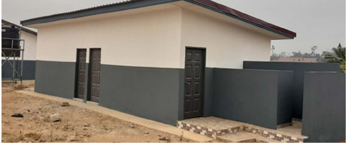
Picture 31 - 1No 10-seater aqua-privy toilet with 2No hand washing facility at New Abirem
