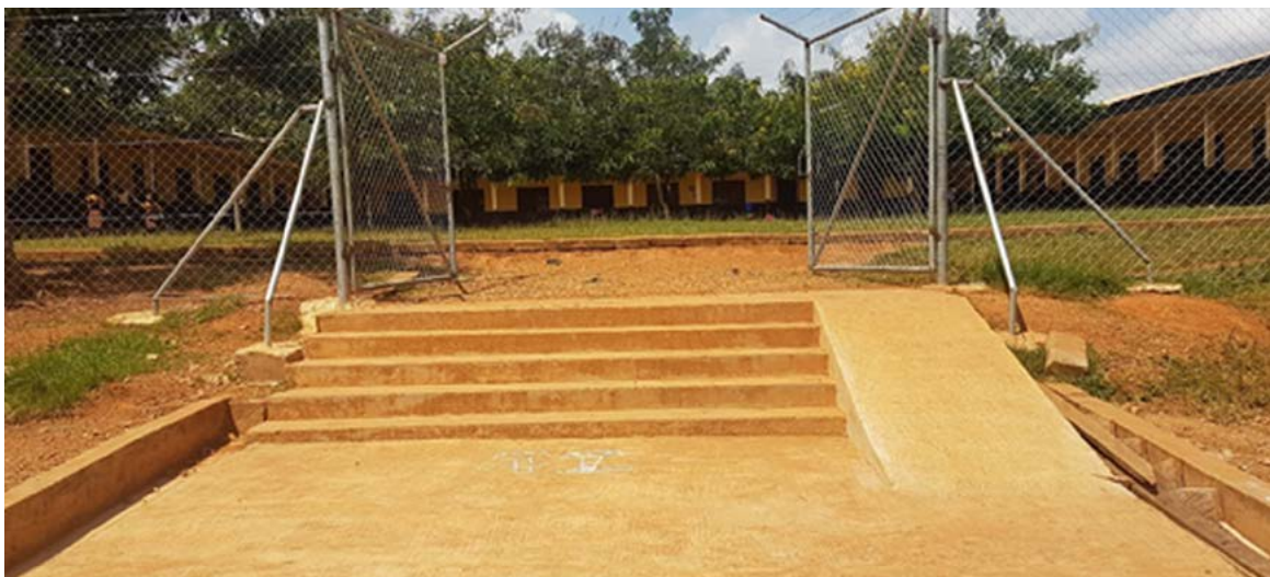
Picture 36 - Chain link Fencing and disability walkway Resettlement Yayaaso DA Basic School
